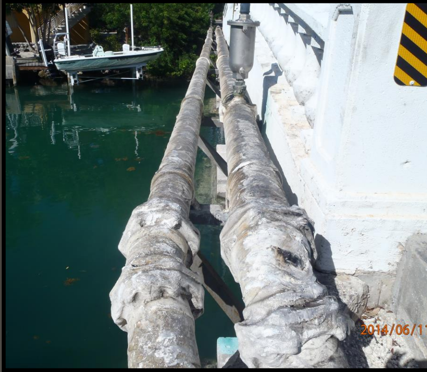
Bridge Mounted Utilities
