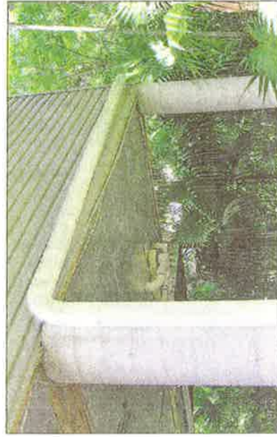
The water is diverted from the downspout to the cistern.
