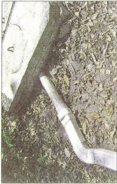
How the gutter feeds into the septic-turned-cistern tank.
