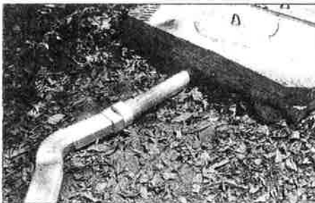
How the gutter feeds into the septic-turned-cistern tank.
